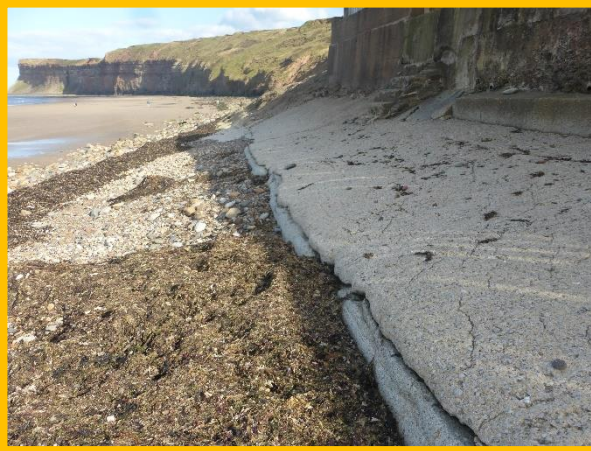
Undercutting of concrete apron (/C0704C05)
