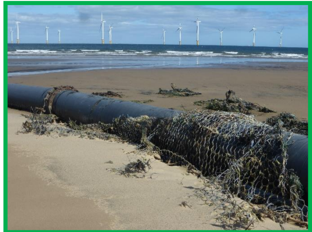
Outfall on Coatham Sands in poor condition (/C0507C01)
