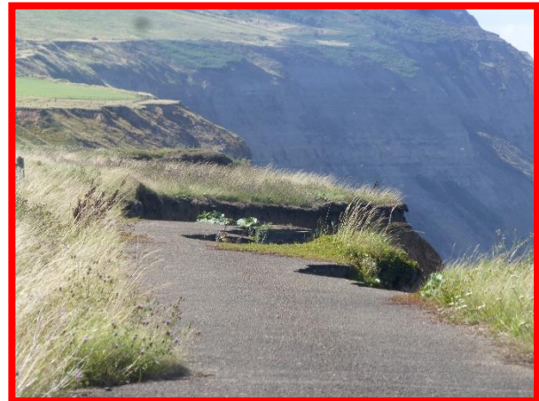
E59/3 Ongoing erosion of soft till layer leading to collapse of road (Totally Active).
