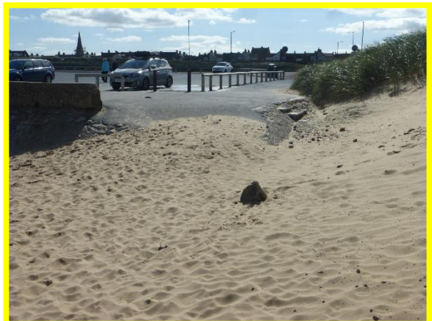
High beach levels have covered previously recorded undercutting of western corner of the asset (/C0601C01)
