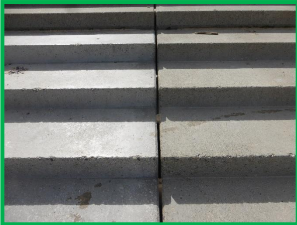
Open joints in stepped concrete revetment. Overall condition remains as very good (/C0602C02)
