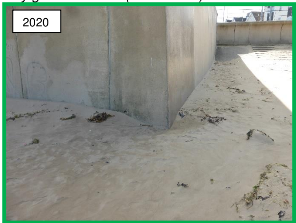
Concrete sea wall at Redcar Beacon note beach levels obscure concrete apron (/C0602C03)
