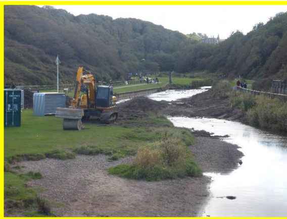
Works ongoing at Skelton Beck, looking upstream from the Saltburn Road bridge.
