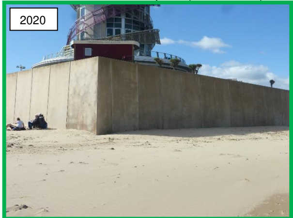
Concrete sea wall at Redcar Beacon note beach levels obscure concrete apron (/C0602C03)
