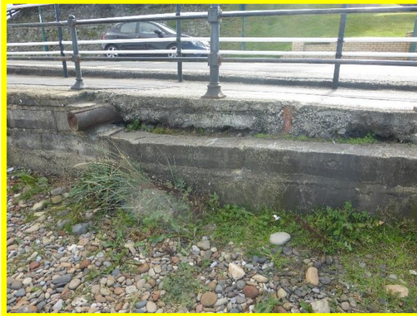
Damage to coping stones along low blockwork wall (/C0704C06)
