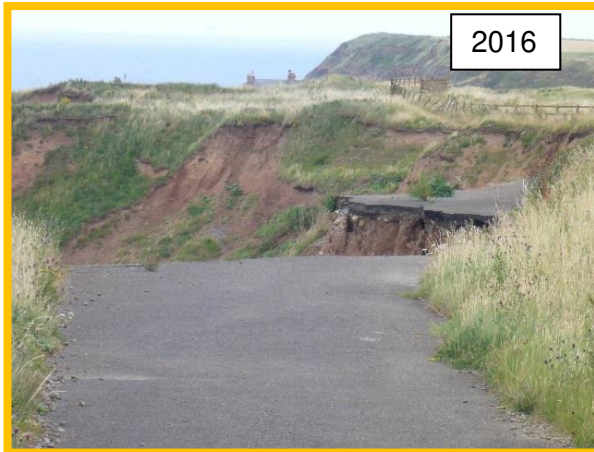
E59/3 and E59/4 Loss of road due to ongoing erosion at Cowbar Lane
