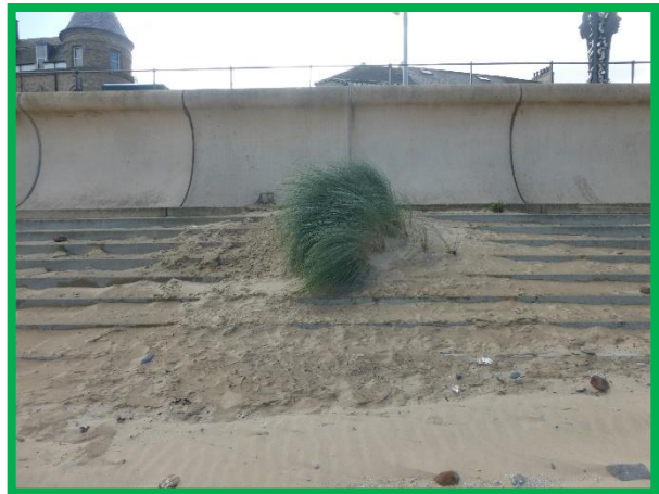
Vegetation growth on stepped revetment. (/C0602C06)
