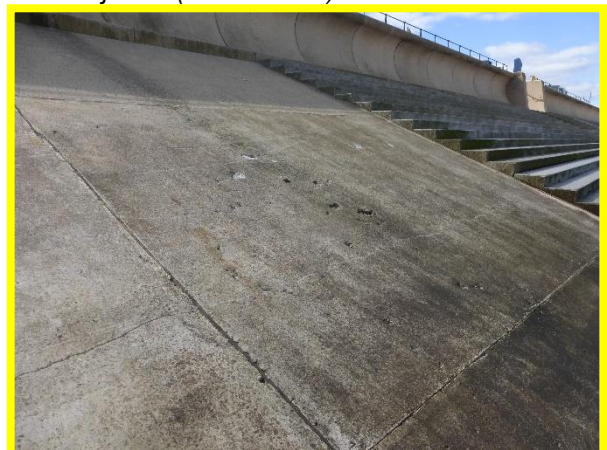
Cracking to mass concrete slabs adjacent to slipway (/C0602C01).
