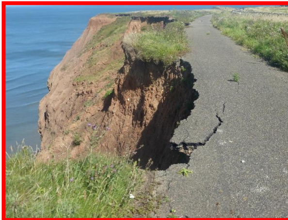
E59/4 Ongoing erosion of soft till layer leading to collapse of road (Totally Active).
