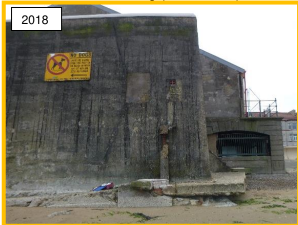
Undercut toe of Cinema seawall visible in 2018 (/C0602C05)
