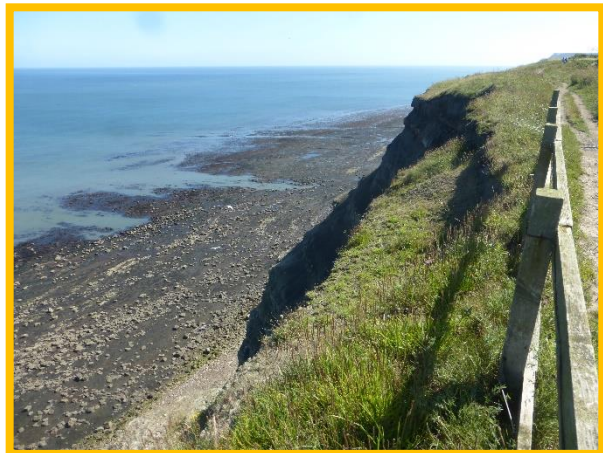
E54/3a proximity of footpath and railway line to actively eroding cliff top (Partly Active)
