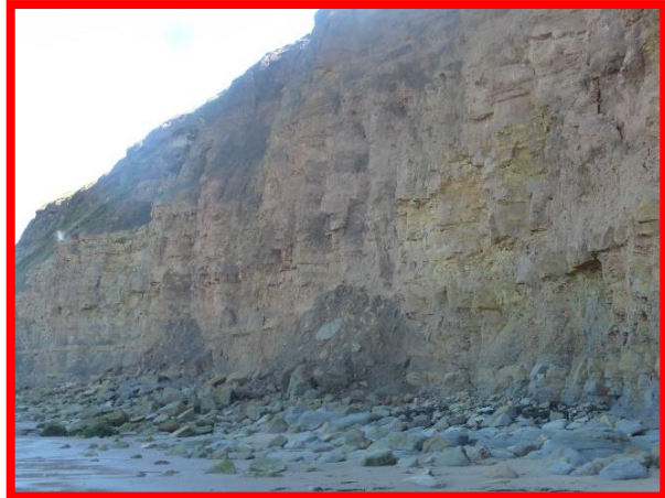
E57/7 evidence of multiple significant rockfalls (Totally Active)
