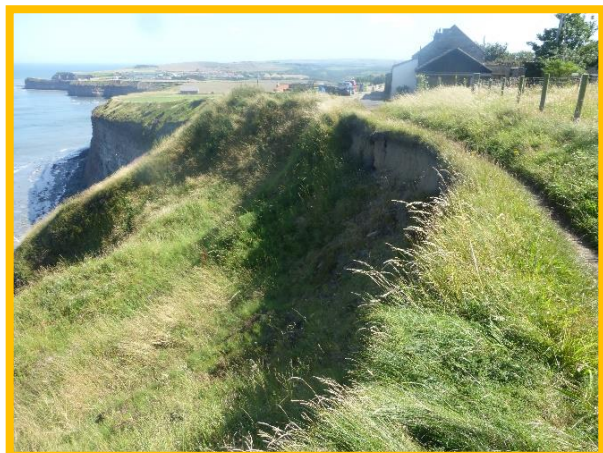
E58/1a headscarp recession encroaching on footpath.
