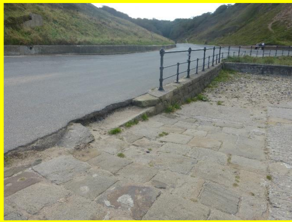
Missing coping stone exposing fill beneath promenade surface (/C0703C02)
