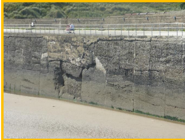
Void visible halfway along inner face of breakwater. (Asset Ref No. 1221D901D0201C02)
