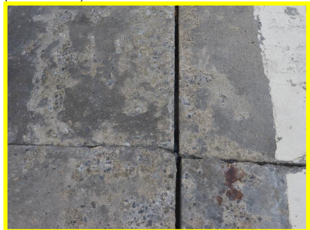
Slipway in fair condition some minor spalling around joints (/C0602C02)
