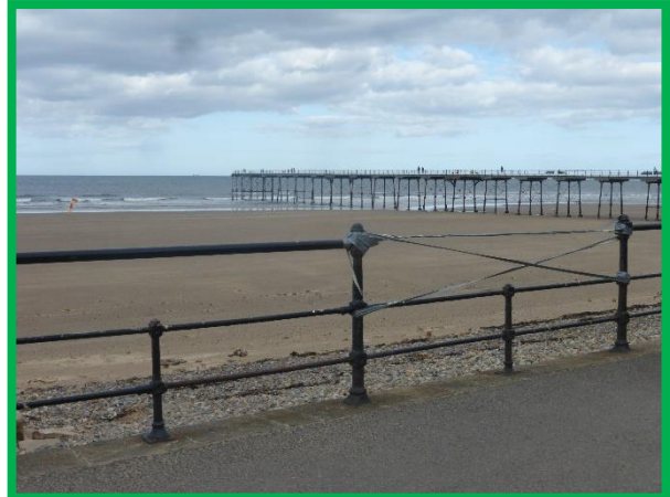
Damage to handrailing along promenade (/C0702C04)
