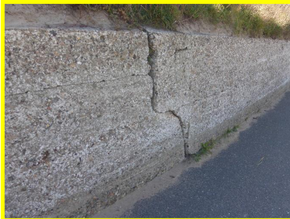
Crack in wall – no apparent change (/C0702C03)
