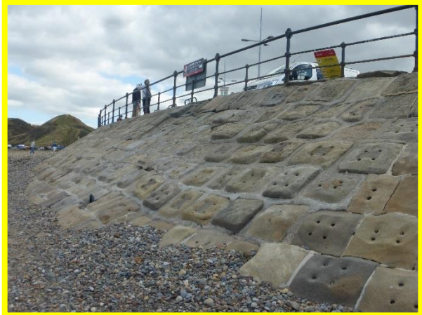
Missing / damaged blocks at apex of structure (/C0704C01)
