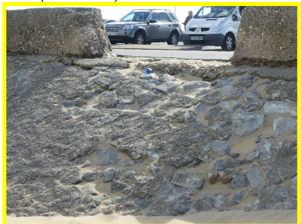
Gap in concrete visible (/C0601C01)
