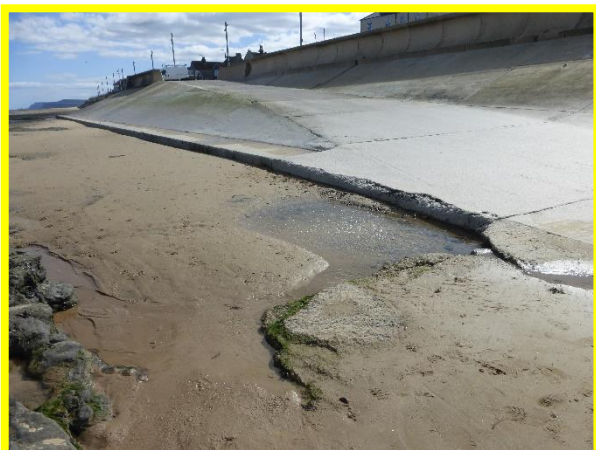
South eastern access ramp. Loss of concrete render exposing grouted stone fill beneath concrete deck slab (/C0602C01).
