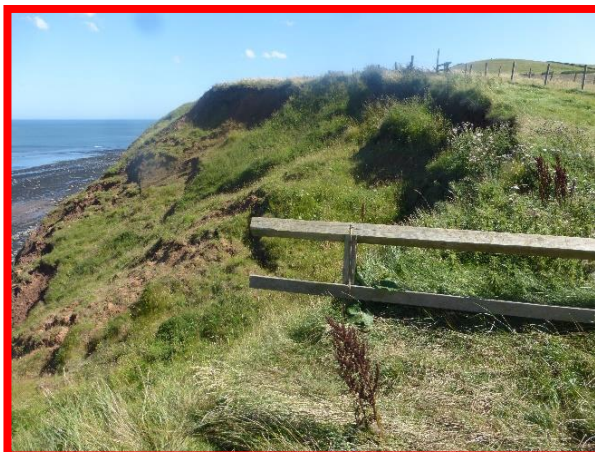
E57/7 Slumping and recession along headscarp (Totally Active)
