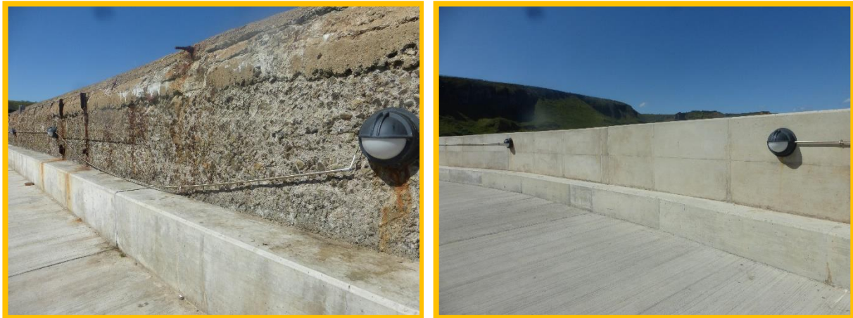
Damaged lighting conduit at head of breakwater. Severed conduit on breakwater.
