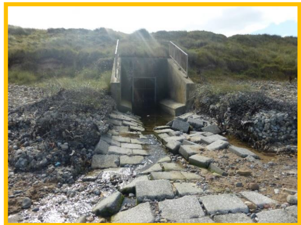
Concrete outfall structure, note failed gabions and scour protection (/C0701C01) CBU E52/10
