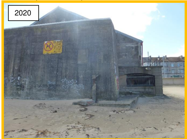
Undercut toe of Cinema seawall buried in 2020 (/C0602C05)
