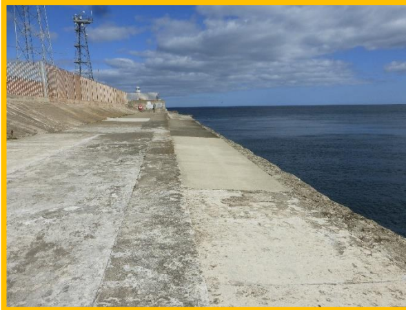
Historic repairs to deck slab along eastern face (/C0506C01)
