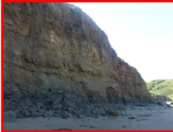
E57/7 evidence of multiple significant rockfalls (Totally Active)
