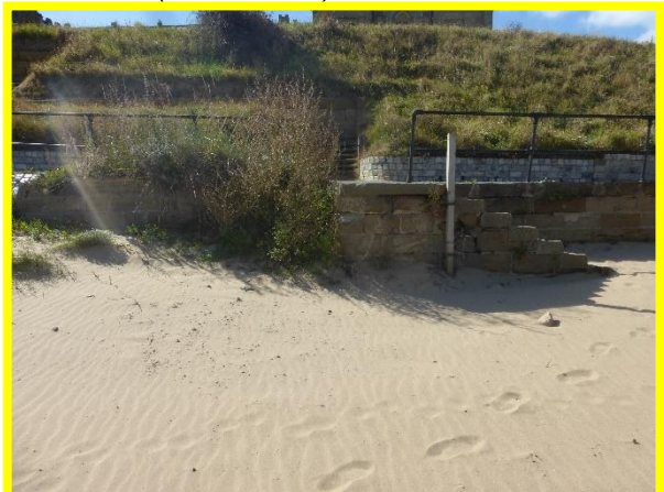
Wall in fair condition some missing mortar and open joints (/C0702C03)
