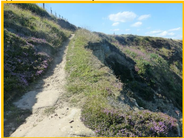
E58/5 Upper further signs of headscarp recession presenting an imminent risk to footpath stability.
