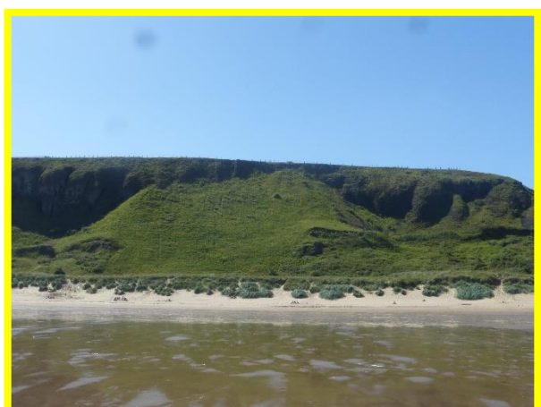
E56/2a and 56/2b Cliffs above Cattersty Sands, looking towards Skinningrove (Locally Active)
