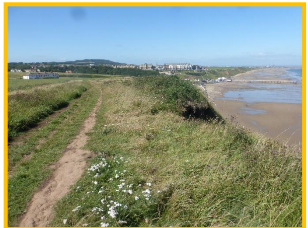
E53/2 Ongoing headscarf recession with some slumping of the till layer of the cliff northeast of Saltburn (Partly Active)
