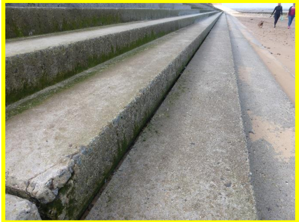
Localized cracking and damage to stepped revetment (/C0602C01).
