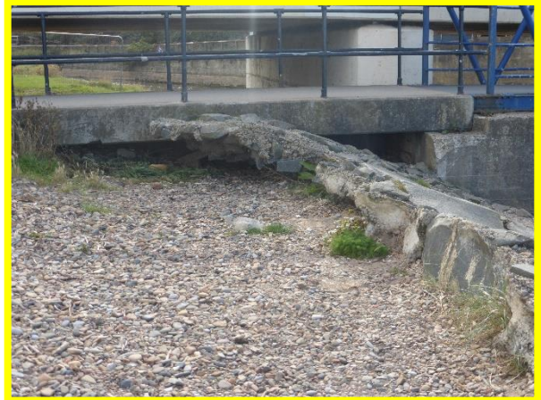
Undercutting of rock revetment apron (/C0704C06)
