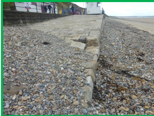
Damage to slipway coping (/C0702C04)
