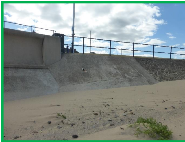
Mass concrete transition in fair condition. Note; horizontal and vertical cracks and damaged drain outfall (/C0602C06)
