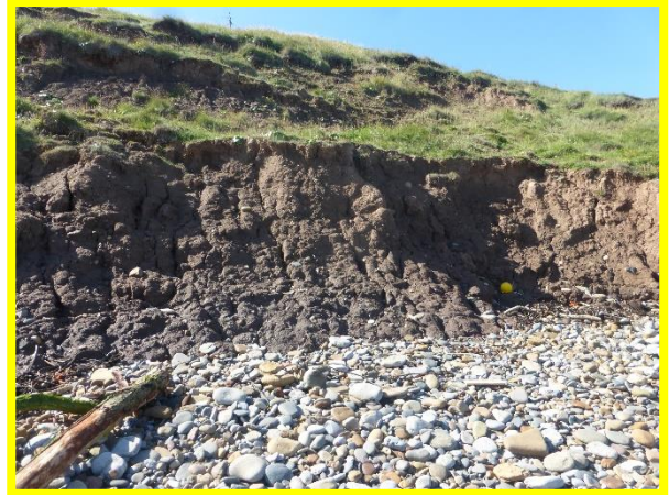
E53/5 ongoing erosion of the toe directly east of Saltburn (Locally Active).
