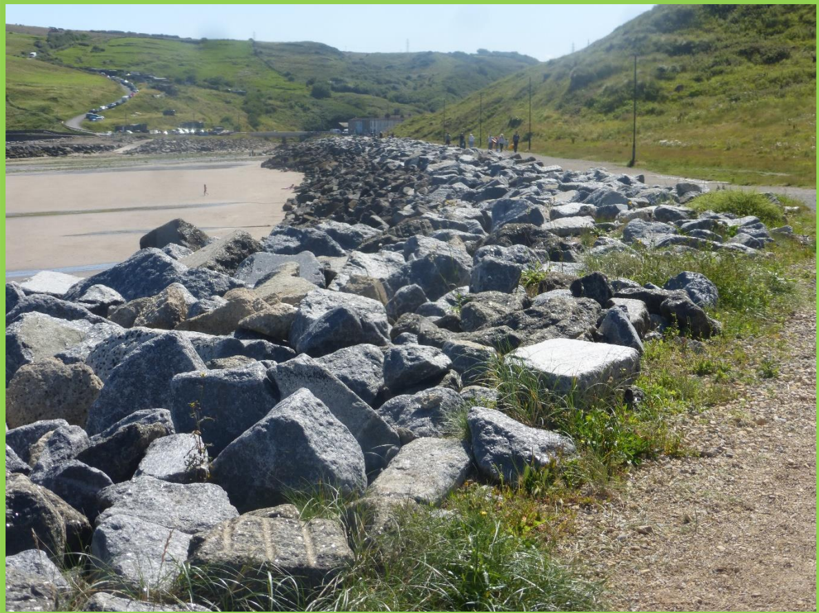
General view of modified revetment and surfaced path looking from Jetty towards village in 2020 (Asset Ref No. 1221D901D0202C01)
