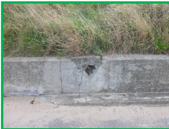
Defects to shallow retaining wall at rear of promenade (/C0702C04)
