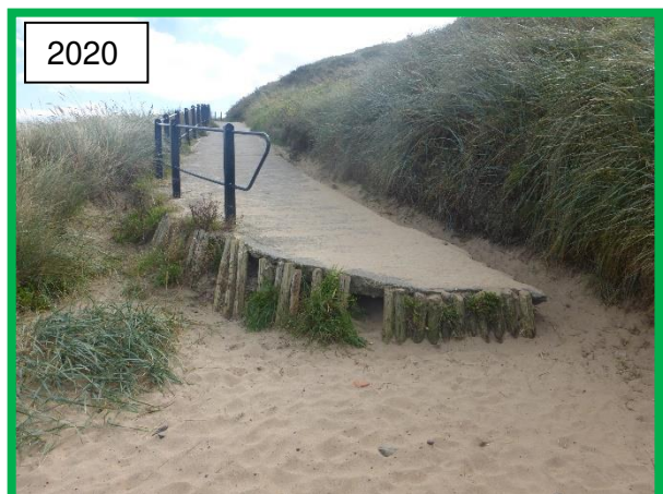
Further exposure of timber piles at foot of concrete footpath (CBU E52/6)
