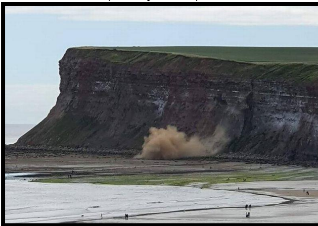
Image of rockfall at E53/2 occurring on 20/07/20 taken from Teesside Gazette website.
