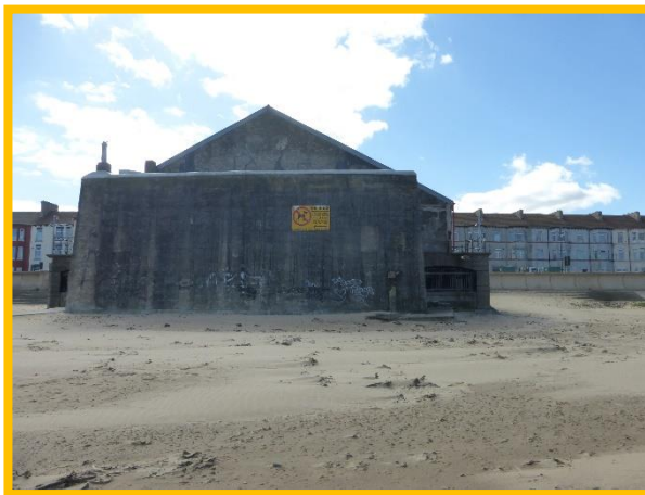
Cinema seawall in poor condition high beach levels cover undercutting (/C0602C05)
