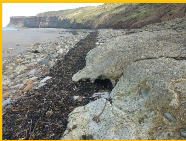
Undercutting of mass concrete apron (/C0704C05)
