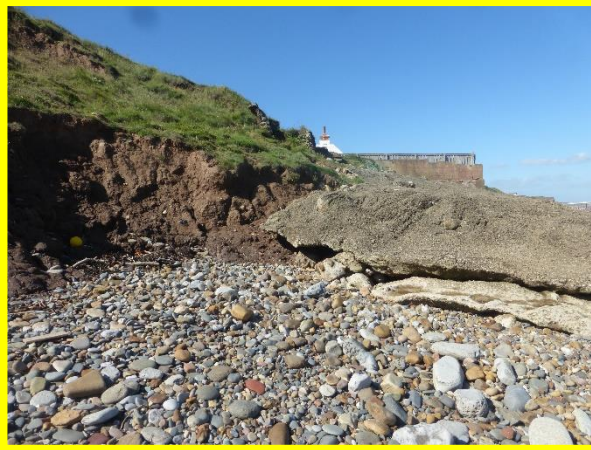
E53/5 Outflanking of the concrete wall at the east end of Saltburn (Locally Active).
