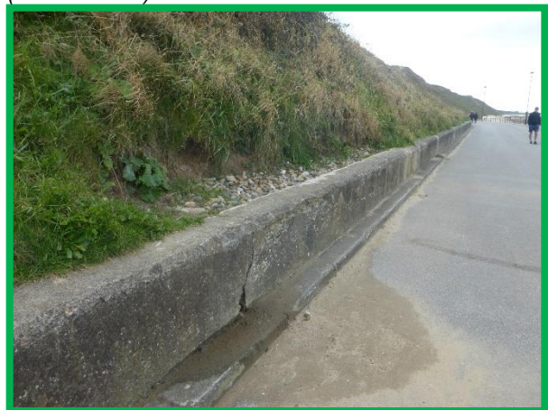
Further damage to shallow retaining wall evidence of material lost from slope to rear (/C0702C04)
