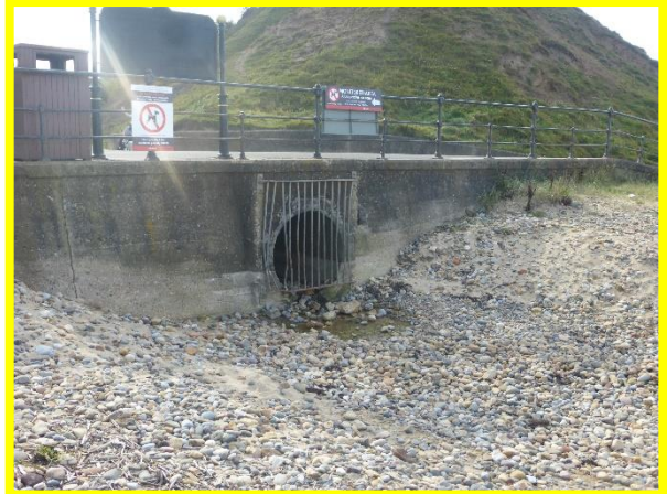
Security grille damaged (/C0703C02). Note accumulation of beach sediment around base of outfall.
