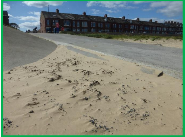
Accumulated sand covers previously noted defects in concrete slipway (/C0602C01)
