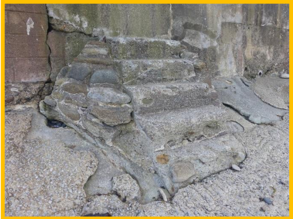
Ad hoc repairs to seawall in poor condition (/C0704C05)
