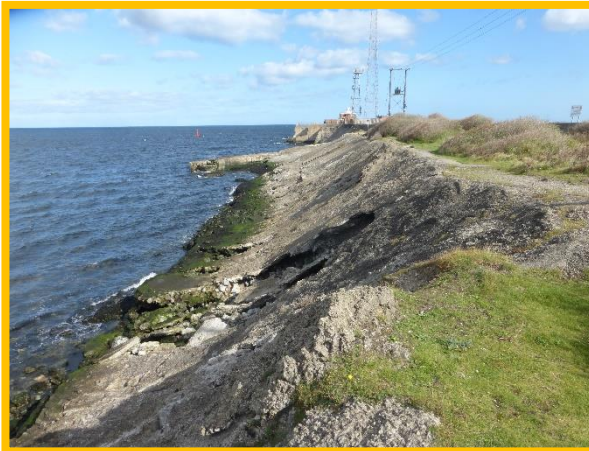
Large void in western face (/C0506C01)
